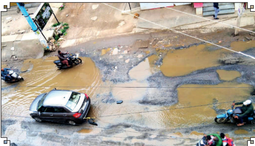
The recently constructed roadways in Anantha Nagara Phase 2 Kamma Sandra are craters with potholes that make it difficult for commuters to navigate.
