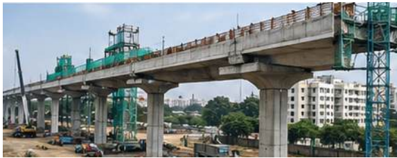
Construction of Bengaluru Suburban Rail Corridor-4 (Kanaka Line) is progressing steadily across key stations including Heelalige, Huskur, Karmelaram, and Bellandur.
